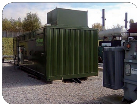
Vykson 140 on a landfill site & grid connected
